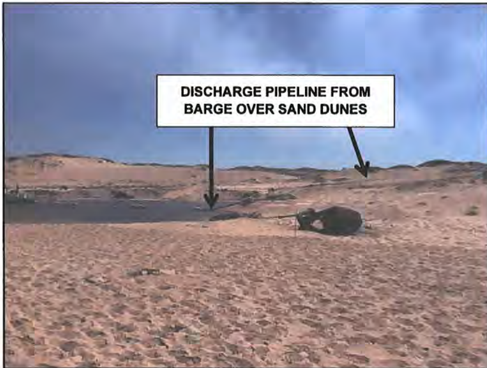
Figure 20 – Dredge Slurry Discharge Line
